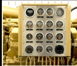
Generator & UPS Inspections
